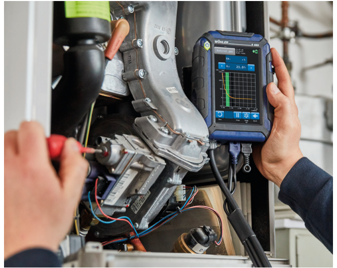
The tuning guide offers an advanced guidance to the technician to properly adjust the burner.
